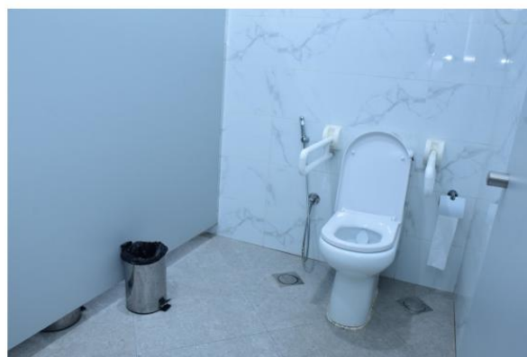
Bathrooms for people with special needs
